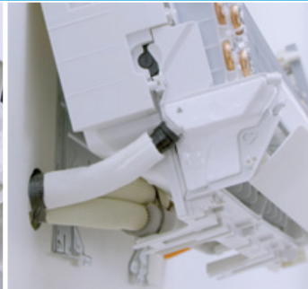
Easy access to drain hose and piping
